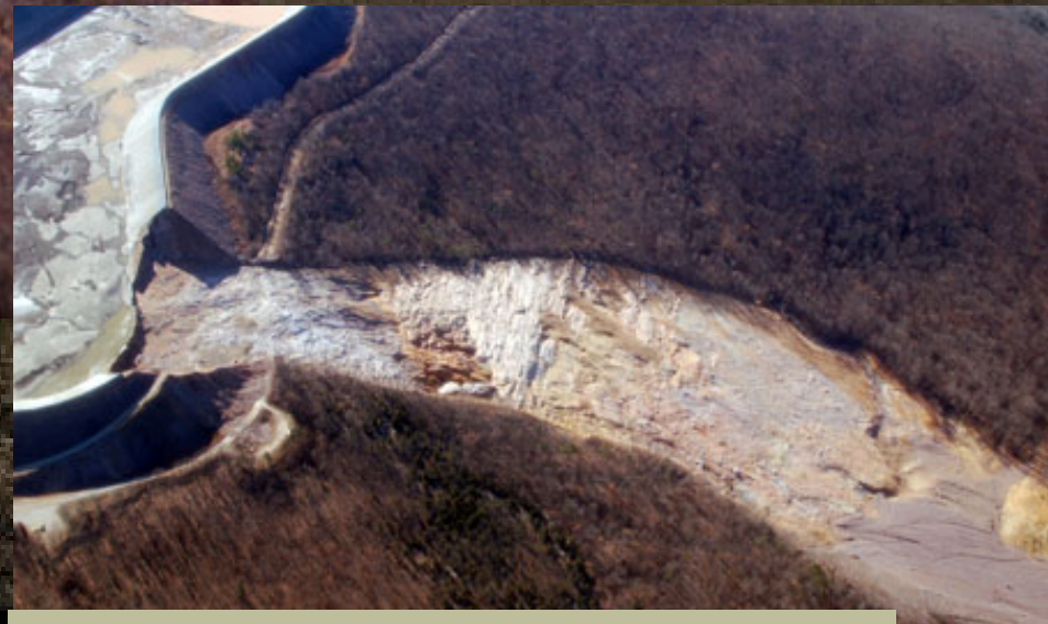
View of breach and scoured surface
