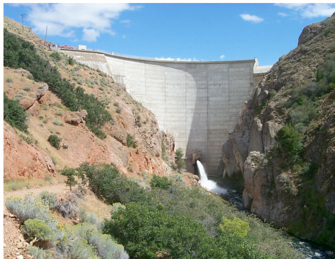
Figure 3. East Canyon Dam. Red truck on far right side of dam (left/right convention relative to looking downstream).
