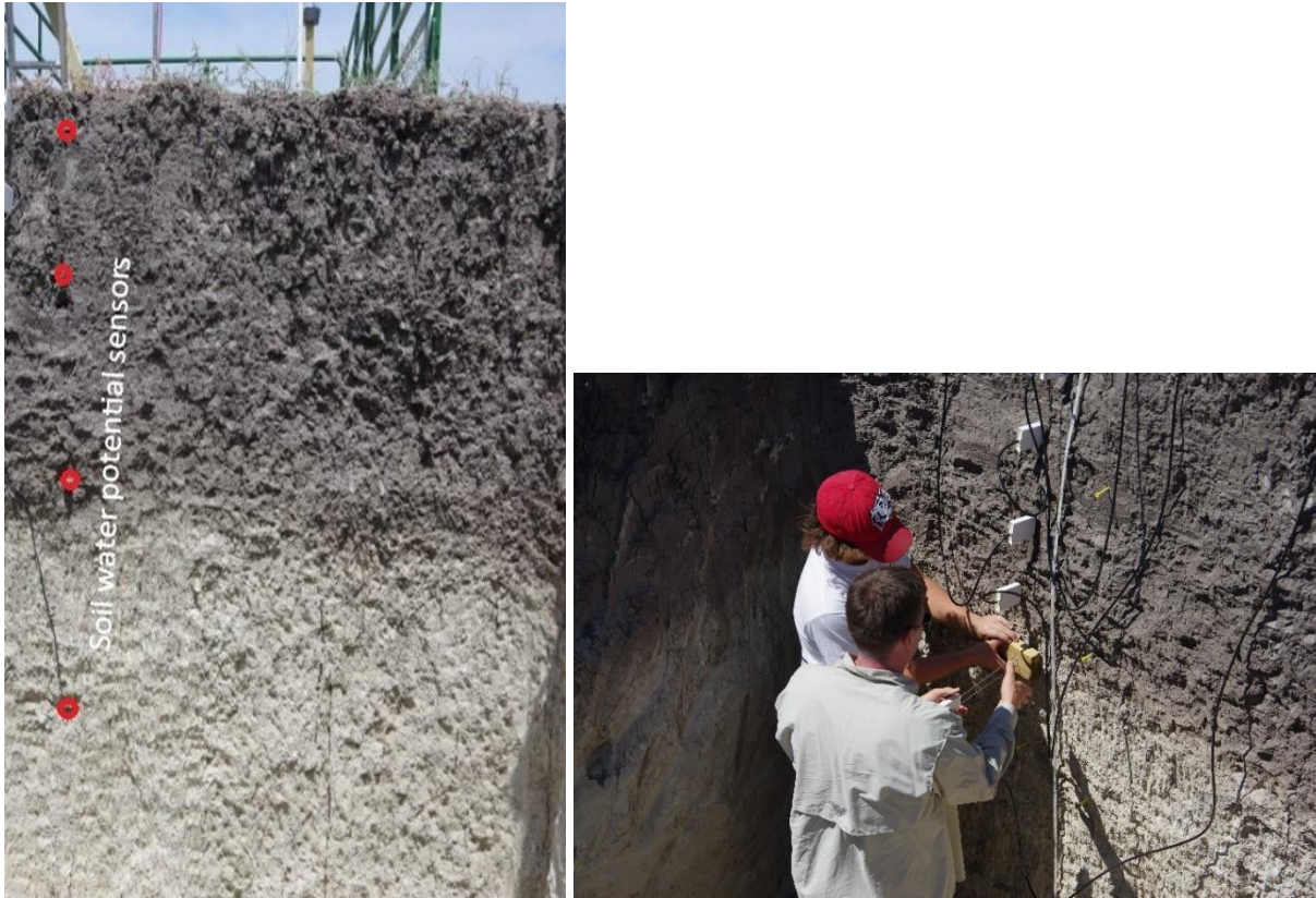
Figure 13. Below-ground sensor installation. (L) soil-water potential sensors emplaced (W.C. Johnson); (R) Dakota Burt (cap) and Randy Stotler installing water content reflectometers. (W.C. Johnson)
