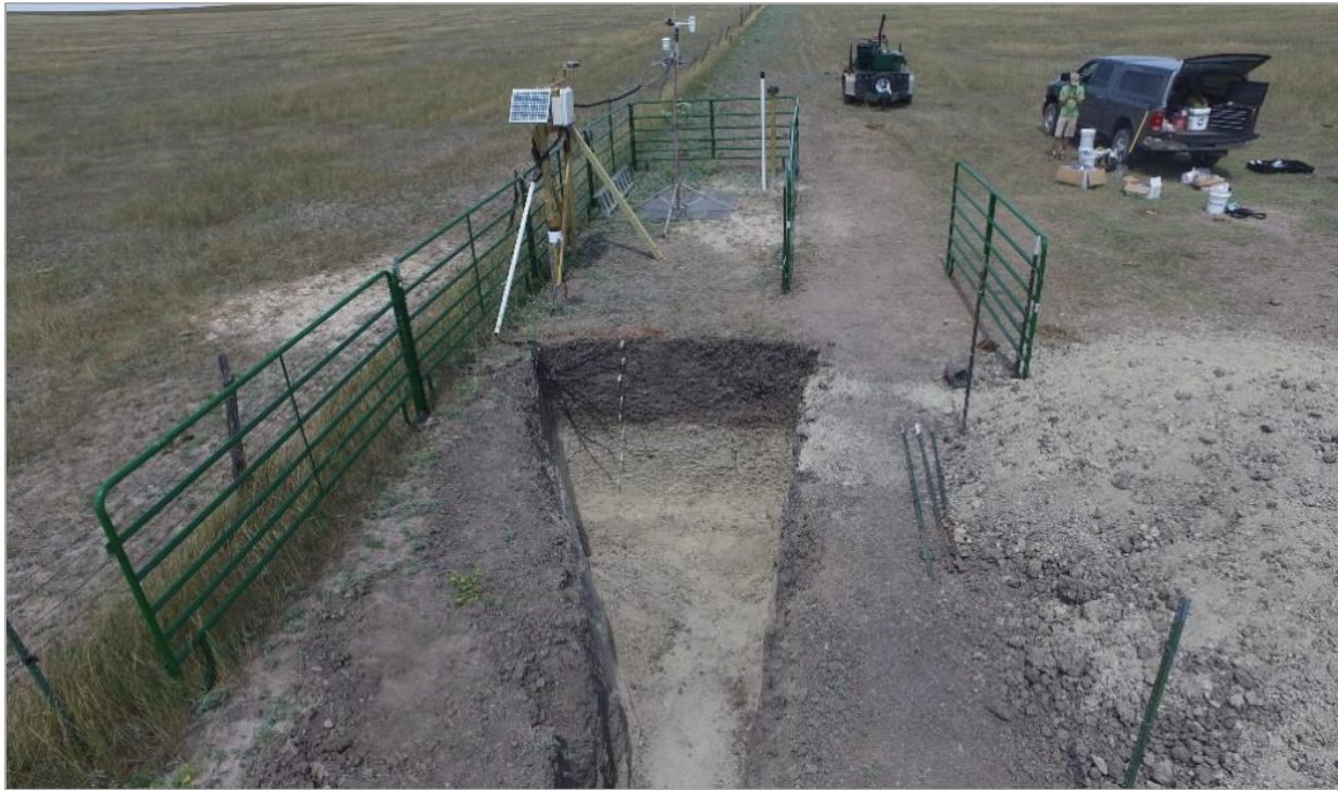
Figure 12. UAS views northwestward of the above-ground instrument array and of the below-ground sensors in the pit prior to backfilling. (D.J. Burt)
