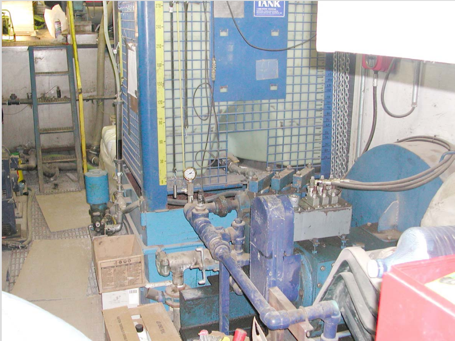
Tri-plex pump and crosslinker storage
