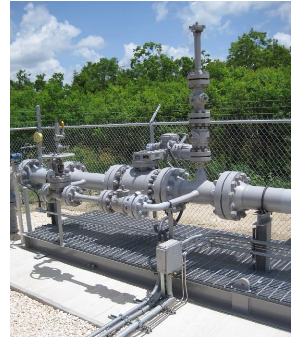
CO 2 Pipeline Meter
