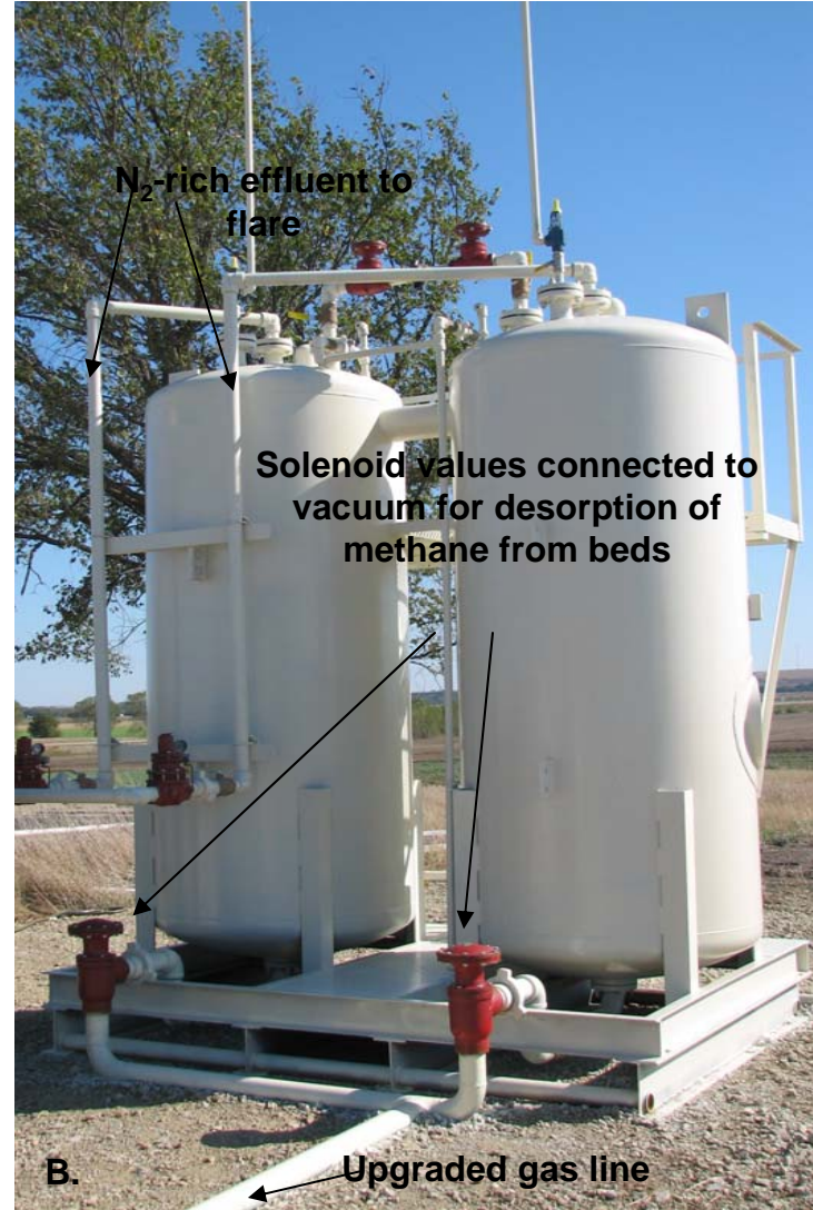
Rear side of the Adsorption/Desorption Towers
