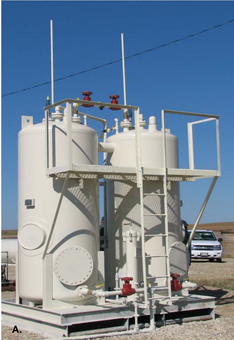
Front side of the Adsorption/Desorption Towers
